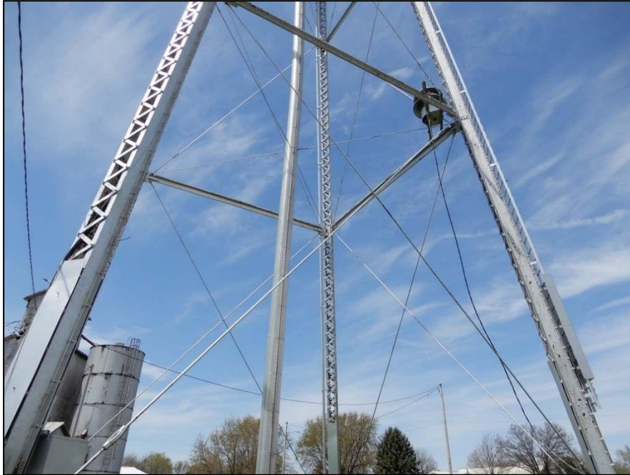
Figure 26. General view of water tower foundation details. Field date of photograph: May 4, 2022.
