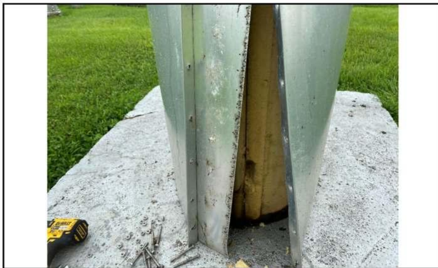
Figure 37. Metal wrapping of insulation on vertical pipe. Source: Viking Industrial Painting 2020:E3.
