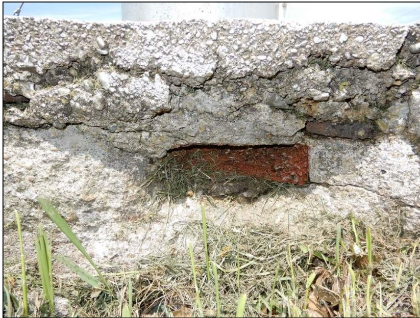
Figure 30. Close up on cement foundation at center of water tower and brick embedded within. Field date of photograph: May 4, 2022.
