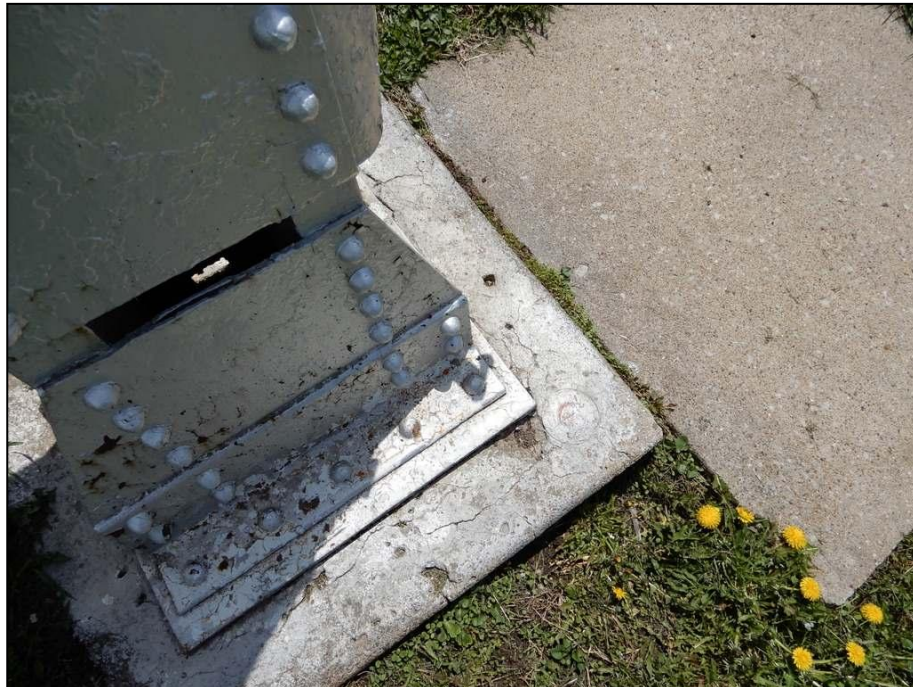
Figure 23. Close-up on base of water tower leg. Field date of photograph: May 4, 2022.
