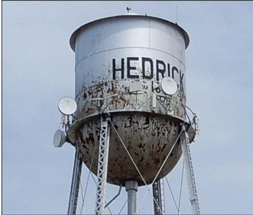
Figure 21. Close-up of water tank showing zig-zag hand railing around base and the cylindrical vent at the roof apex. Field date of photograph: May 4, 2022.
