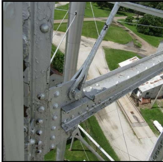
Figure 34. Northeast leg, looking south. Upper strut joint with angled rod and leg. Source: Viking Industrial Painting 2020:5.
