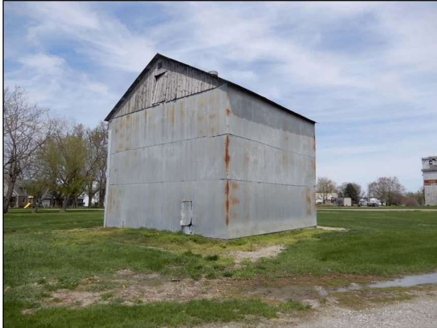
Figure 13. Facing NW towards building near proposed water tower area. Field date of photograph: May 4, 2022.
