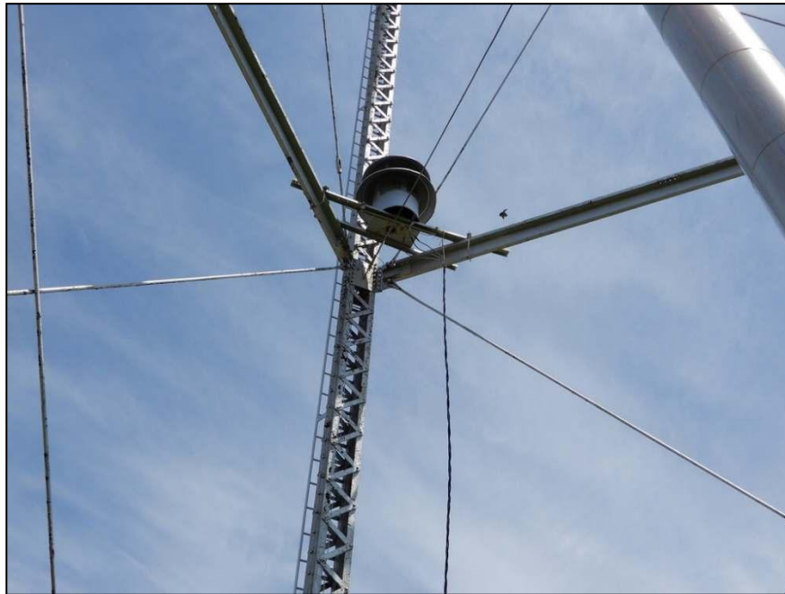
Figure 28. General view of water tower joint details and city siren. Field date of photograph: May 4, 2022.
